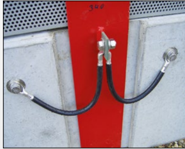
earthing terminals at base elements
